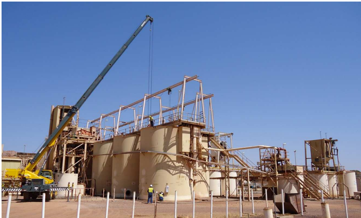
1Mtpa nameplate Grosvenor gold plant
